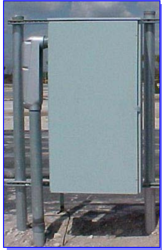
NEMA 3R enclosure containing a 400A. Company Switch outside the Orange County Convention Center in Orlando, FL. The 400A. Company Switch is completely enclosed and protected from weather and vandalism. The cable entry trapdoor on the bottom of the enclosure is closed and locked
